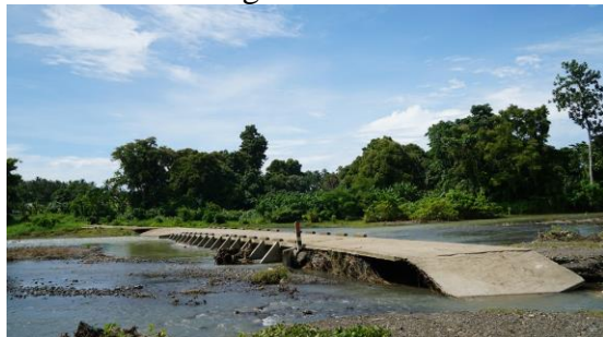
Photo 2: A damaged bridge
