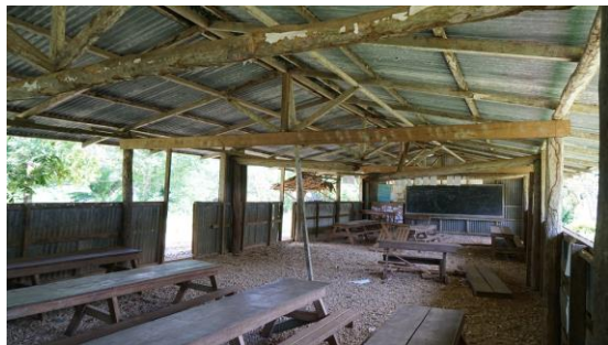
Photo 1: A damaged school – will not be open in time for the 2017 school year.
